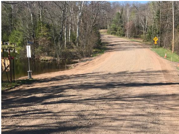
Diamond Lake boat launch May 20, 2020. Grading has been improved from earlier in the year to reduce the slope into the water. It's quite reasonable now but still soft. Pioneer Rd. has been graveled in both directions for about 400 yards as part of the new culvert project, pavement is anticipated sometime in summer 2020.
