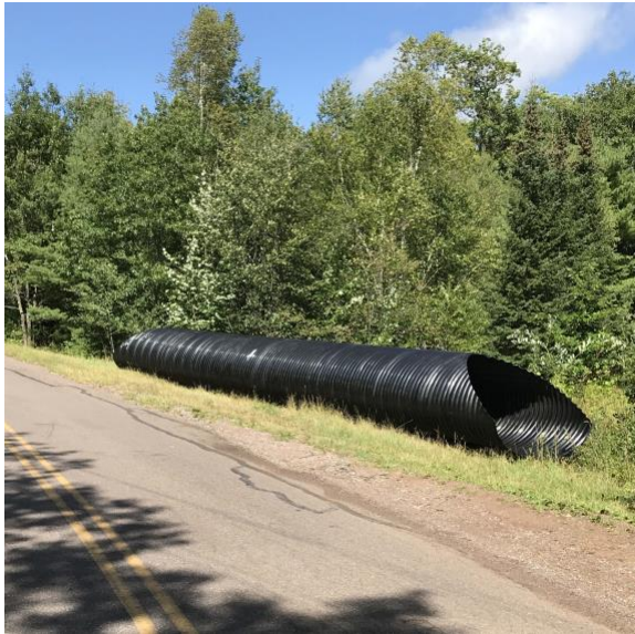
Long Enough? The new 5 foot diameter culvert ready to be installed beneath/ across Pioneer Rd. near our boat launch. This will replace the much smaller diameter pipe that currently brings the outflow from Crystal Lake into Diamond and (hopefully) accommodate larger rain events in the future. -RJ
