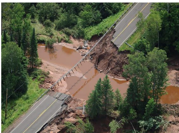
Hwy 169 in Iron County after the July 2016 Storm. Wisconsin Emergency Management photo.
